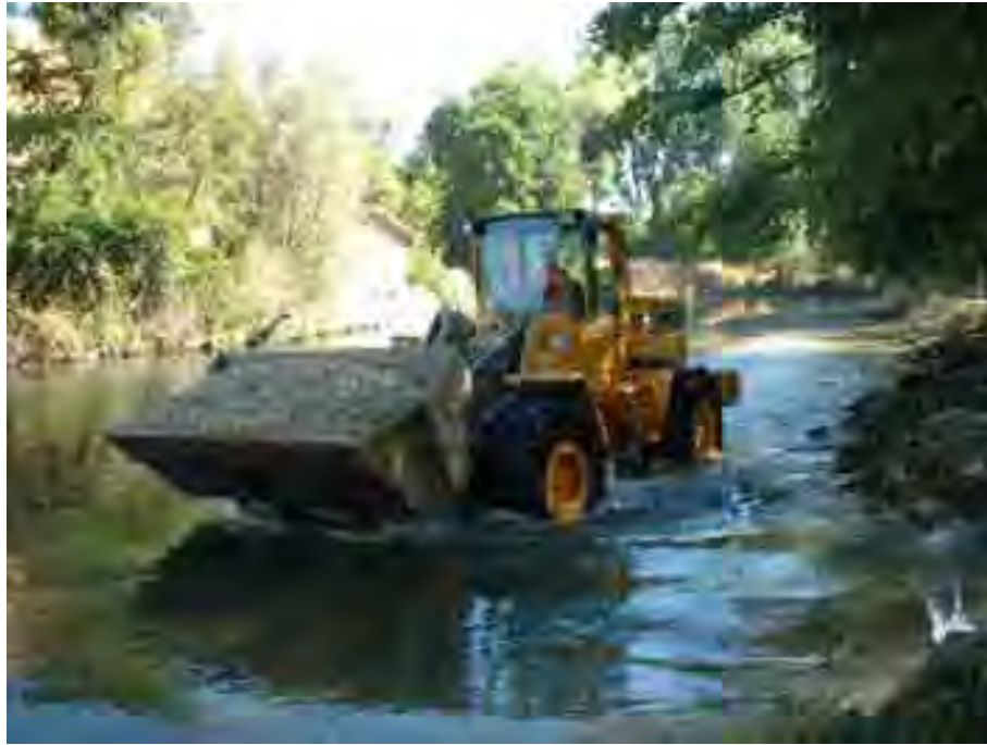
FIGURE 1.1: Despite all the rhetoric calling for 'catchment-scale restoration', most PHR involves active intervention (i.e. construction of habitat features) at the reach scale as shown here. In this case gravel is being placed in a channel downstream of a dam to construct riffle and bar habitats for salmon. Photo from PHR in 2001 on the Mokelumne River, California (photo by Author).
